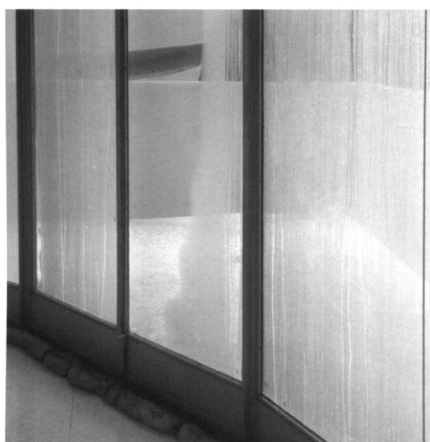
Fig. 2. Seasonal condensation at original fourth-floor interior steel-frame glass walls, photograph 2005. This and all other photographs by Angel Ayón, WASA/Studio A, unless otherwise noted.
